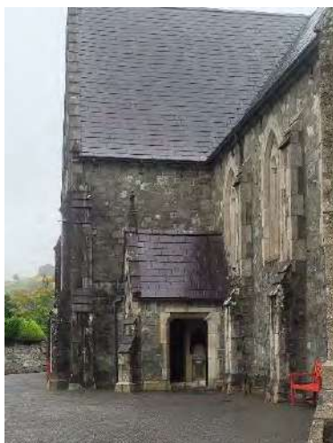
North west entrance porch presently main entrance; view south of west transept. Few slipped slates noted to high level roof.
