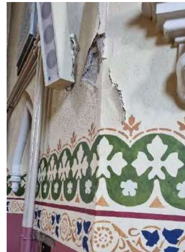
Section of cracked and boasted plaster at the junction between the nave and east transept.
