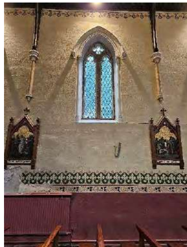
Window W-G13, fixed window. Loss of stencilled paintwork detail and boasted plaster below cill level. Plaster repairs apparent at low level.
