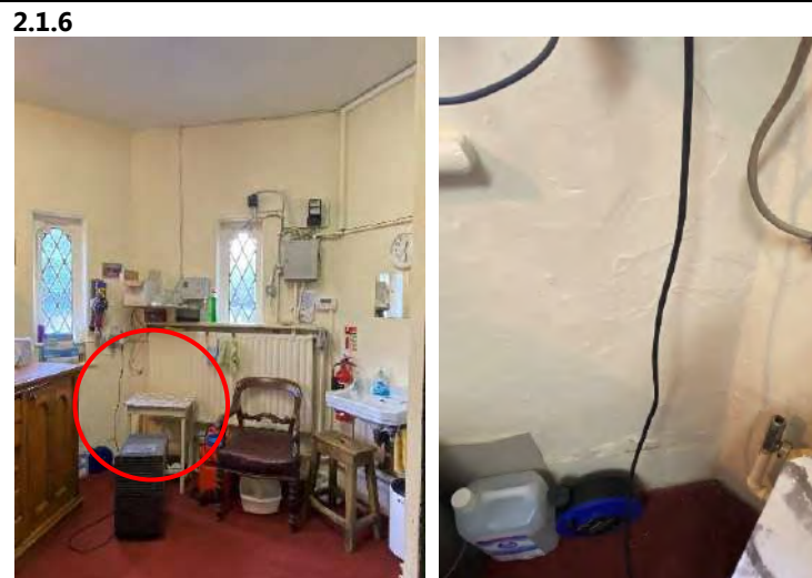
View towards north wall of the sacristy, below window WDW-G03 patches of previously repaired boasted plasterwork. Note ESB meter.
