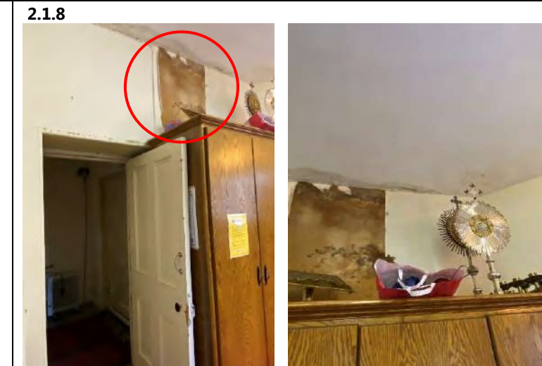
View south east towards door G-D02. Section of active dry rot visible at high level. Staining to wall and ceiling in this location.
