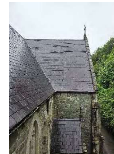
South pitch of East Transept Roof. Roof A, pitch A8 and Roof E, pitch E1 (to entrance lobby). Some localised slipped slates.
