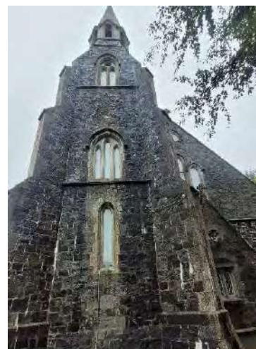
Bell tower; south elevation; central view. Secondary storm glazing to windows. Lime leaching to stone.
