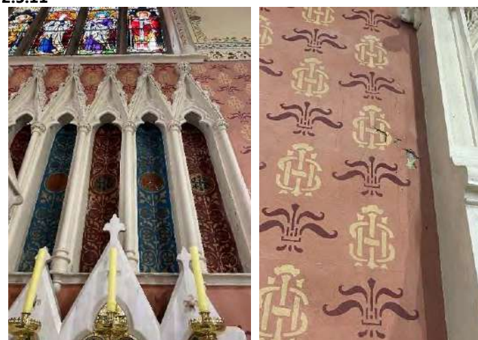
View of the niches behind the alter including small localised areas of boasting to the plasterwork which has been stencilled.
