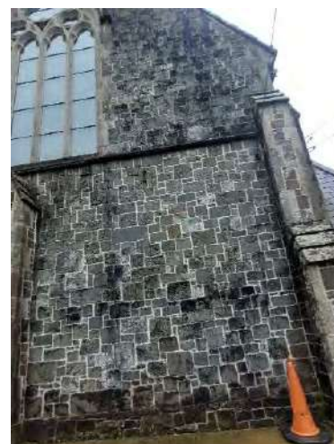
North elevation behind Altar: right hand side. Façade re-pointed. Staining at low level likely due to rising damp.
