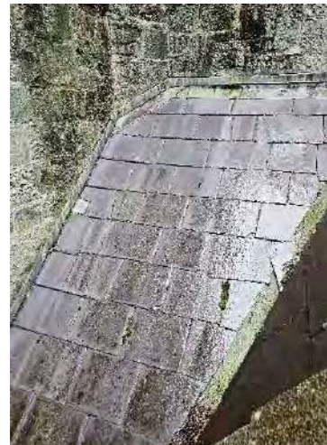
Roof G to the south porch in poor condition; broken and slipped slates, algae growth, minimal lead flashing against stone wall.
