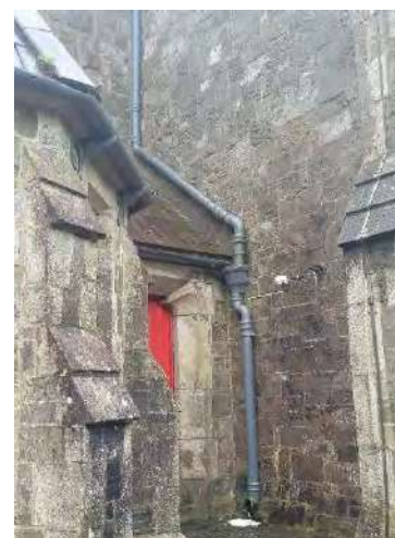
Rainwater pipe RWP-10 in poor condition with overflowing gully. North elevation along west transept with entrance door to sacristy.
