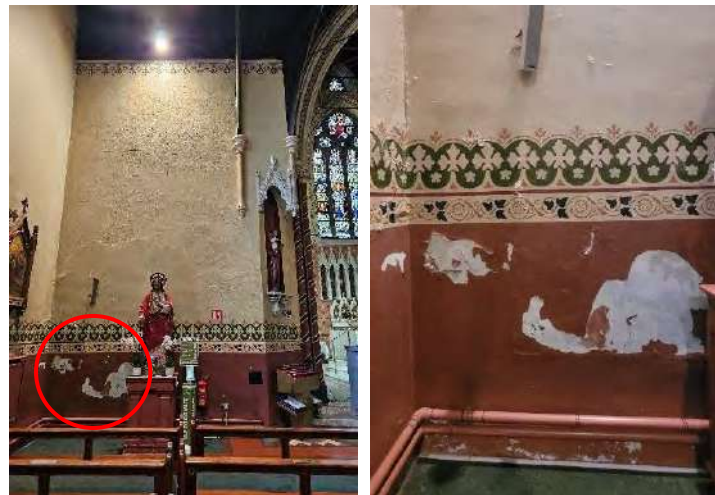
North wall view of the west transept in poor condition. Missing paintwork and boasted plaster. Areas has been partially replastered.
