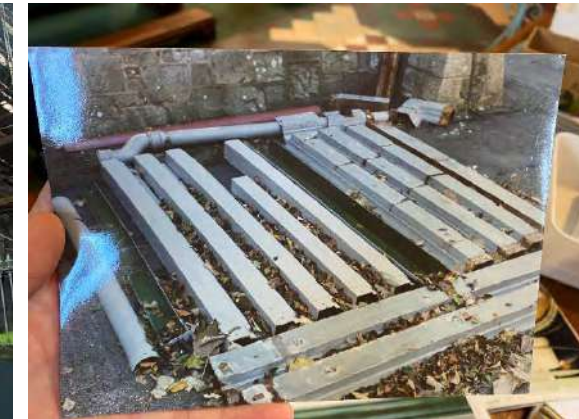
Fig 11: External photo of Avoca Church, rainwater goods, assumed 2000, provided by Fr Michal Murphy P.P.
