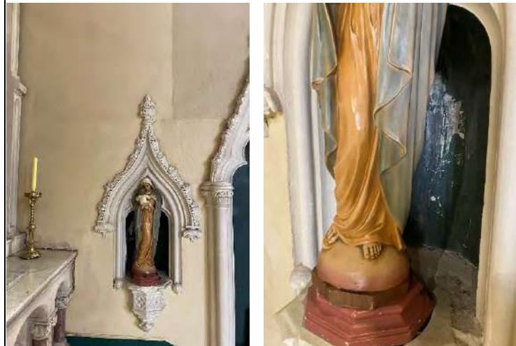
Detailed view of decorative statue niches. Entire niche has boast plaster. Three remaining niches have tide lines and efflorescence.
