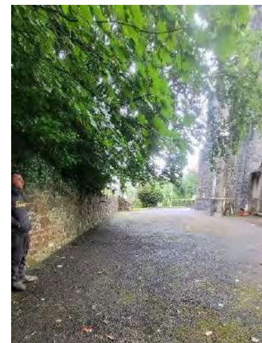
South boundary wall. Heavy vegetation growth.
