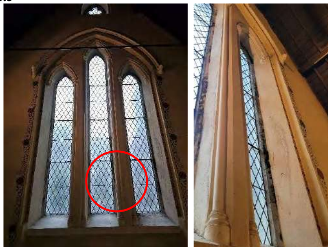
View of window W-G27 to choir balcony. Heavy mould growth to the stone mullions and water staining to painted reveals.
