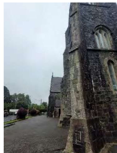
Bell tower; south elevation. Heavy staining and lime leaching to stone. Tarmac surface throughout.
