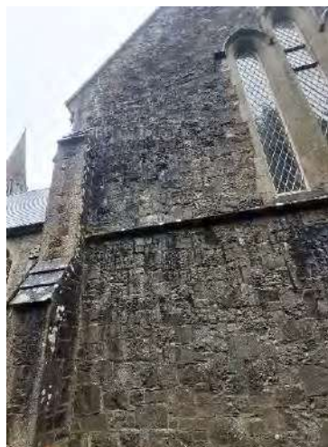
East transept; left hand side. Heavy staining and cementitious pointing to stone.
