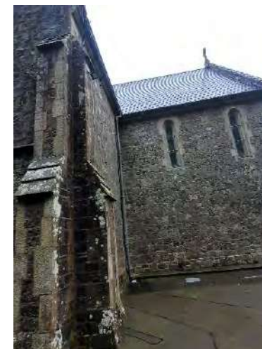
East wall of Alter. Windows W-G07 & W-G06 at high level. Heavy algae growth to ground surface due to water ponding.
