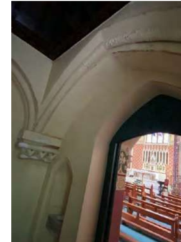
View north west including door D-G04. Paint and plaster finishes deteriorated, corrosion of metal beading apparent to head of door.
