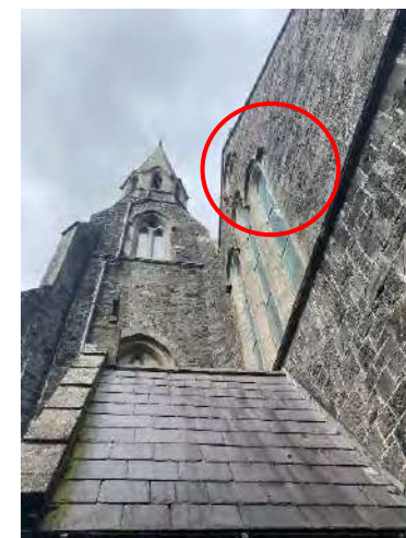
South elevation. Roof F, pitch F2. Note vegetation growth to window W-G27 and secondary storm glazing to exterior face. Lead flashing minimal to roof junction.
