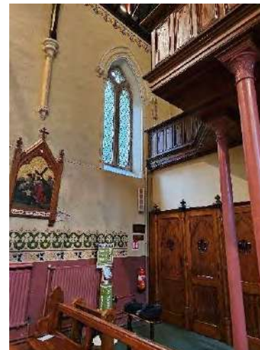
Window W-G15, fixed window. Boasted plaster below cill level. Plaster repairs apparent at low level.
