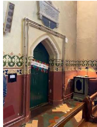
View of door G-D12 including piped services surrounding. Plasterwork in poor condition at low level.
