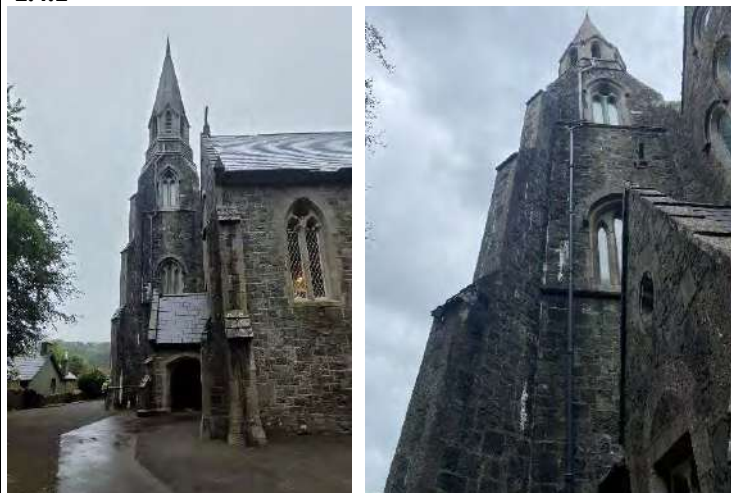
Bell tower view east. Entrance via south porch. Staining and lime leaching to stone. Extended rainwater pipe to top of tower. Secondary storm glass to bell tower windows.
