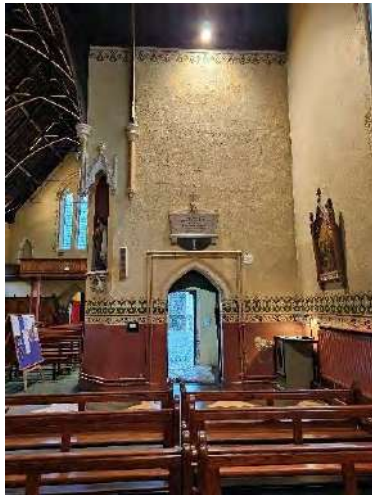
View south of door G-D12, west transept. Plasterwork in poor condition.
