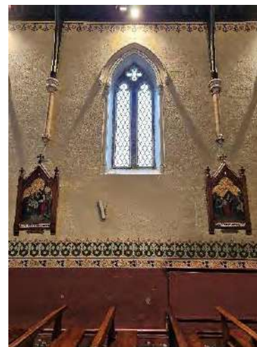
Window W-G21. Note boasted plaster below cill level. Fixed window.
