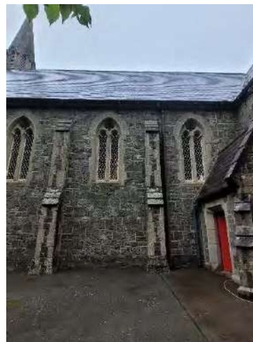
Windows W-G12 & W-G13. Entrance to north east porch. Tarmac surface throughout which has algae staining due to water ponding.
