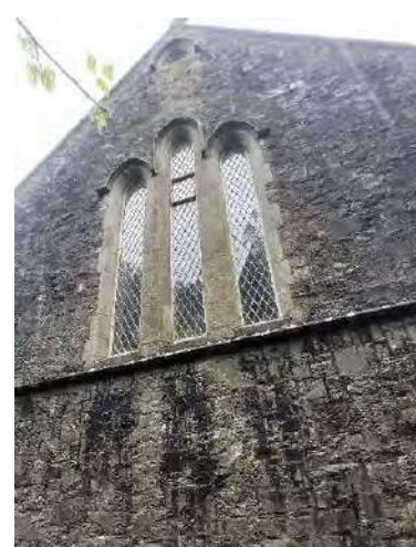
East transept; view centrally. Heavy staining and cementitious pointing to stone. Operable section of window not operational.
