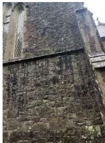
East transept; right hand side. Heavy staining and cementitious pointing to stone.
