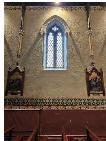
Window W-G20. Note boasted plaster below cill level. Fixed window.
