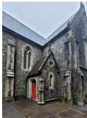
North east entrance porch. Heavy staining to stone.
