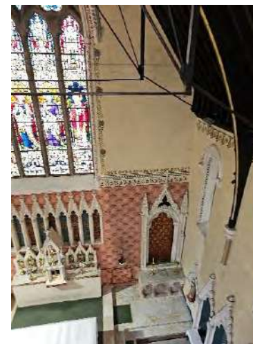
High level view of the alter rhs. Small localised area of boasted plasterwork at high level. Lined-and-ruled plaster finish.
