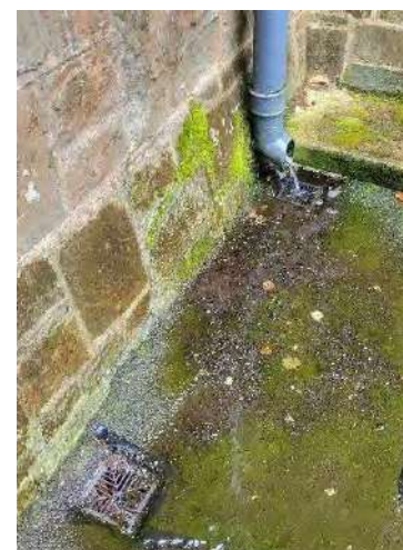
Algae growth around rainwater gully to RWP-07. Gully overflowing.
