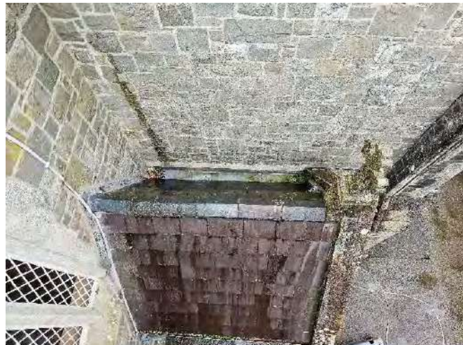
Valley gutter and roof E, pitch E2, to north east entrance porch in poor condition.
