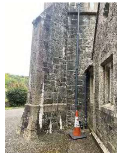
Lime leaching to snecked rubble stone at bell tower on east elevation. Gulleys overflowing and algae growth to tarmac surface.
