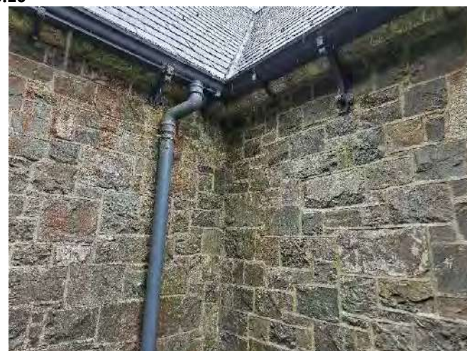
Rainwater pipe RWP-07. Algae growth apparent to high-level stone band supporting gutter.
