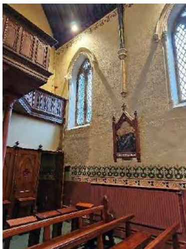
View south west, window W-G19. Note boasted plaster below cill level.
