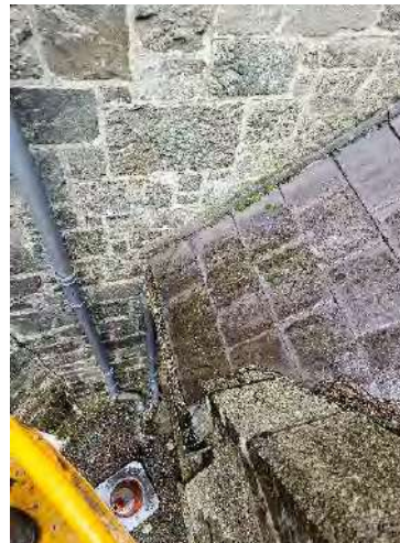
RWP-01 and RWP-02 to the bell tower and Roof G. Cast iron gutter blocked and causing staining to slated roof.
