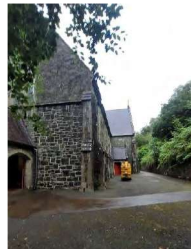
North east entrance porch; view south of east transept. Tarmac surface throughout with algae growth.
