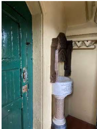
View north east towards door G-D12. Base of door and reveal showing signs of damp due to water ingress.
