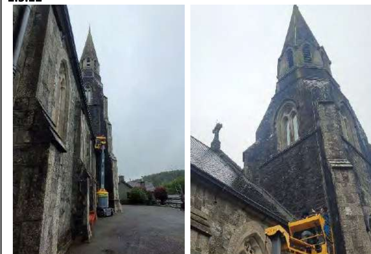
North elevation of the bell tower. Heavy staining and localised lime leaching to stone. Secondary storm glazing to windows.
