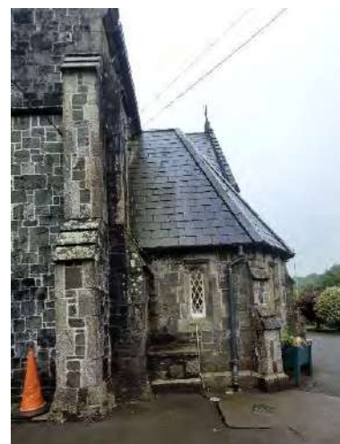
Sacristy, windows W-G04. Rainwater goods in this location are poor functioning.
