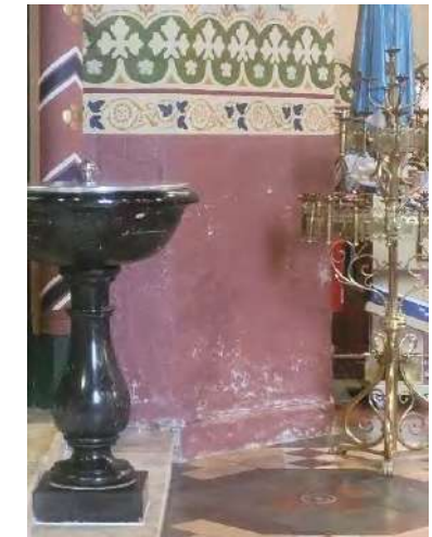
View of junction between the altar and the north wall of the east transept. Note modern replacement baptismal font and loss of detail to the plasterwork at low level due to repairs and rising damp.
