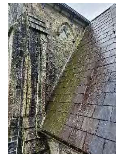
Algae growth to Roof D, pitch D5 along east wall. Staining to stone. Electrical incoming supply seen to buttress entering sacristy.
