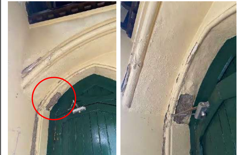
View north west to left hand side of door G-D12. Paint and plaster finishes deteriorated, corresponding with defect to gutter over.
