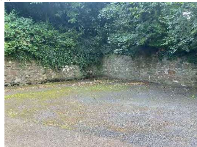
South-east corner of boundary wall. Tarmac surface throughout with aglae growth due to ponding water in this location.
