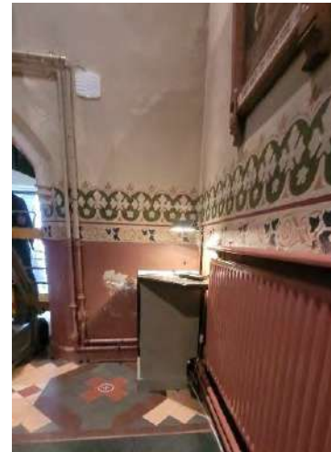
Area of deteriorated plaster finish to the rhs of door G-D12.
