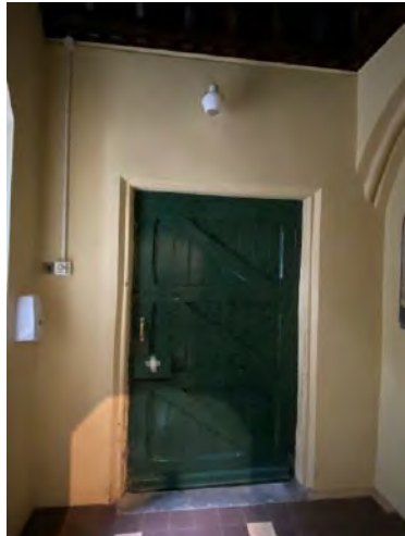
View south towards external door G-D05. Dry lining to this area. Base of door and reveal show sign of damp.
